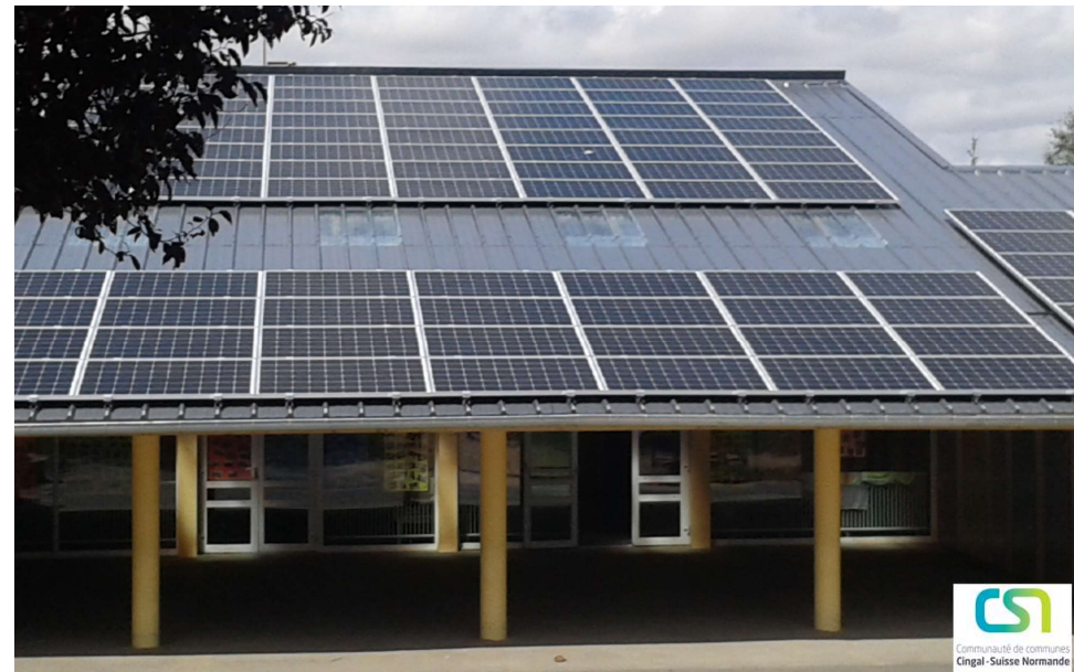
Installation Photovoltaïque de 72 kWc
