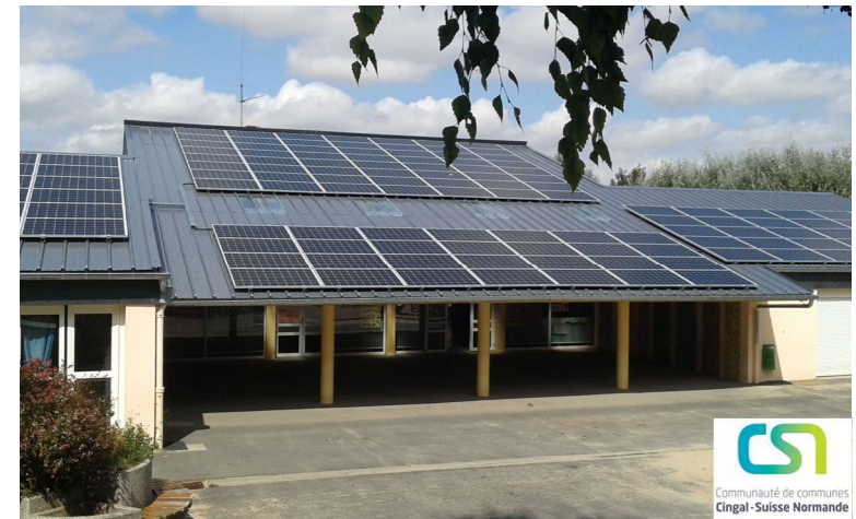
Installation Photovoltaïque de 28 kWc
